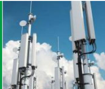
5G Base Station
